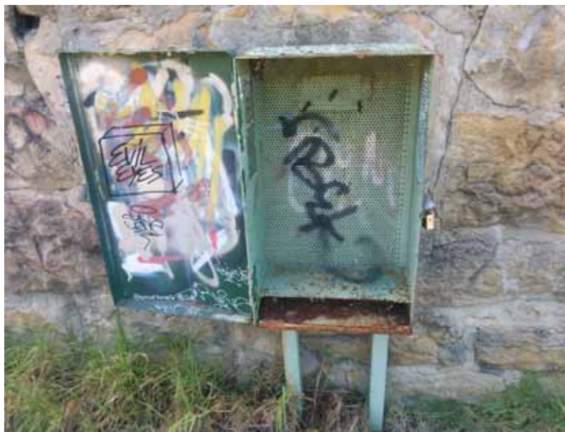
Photo 6 – Electrical box on lower bowling green
