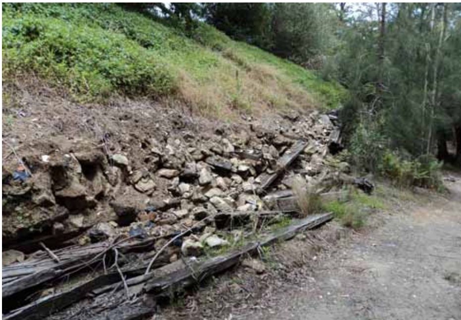
Photo 4 – Damaged timber retaining structures
