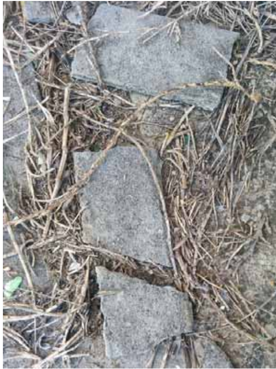
Photo 11 – Potential Asbestos Containing Material
