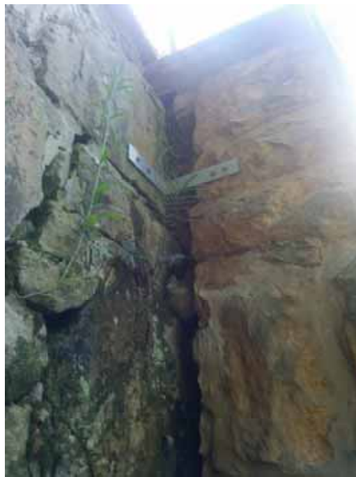
Photo 5 – Failing retaining wall for bowling greens (note metal brace)
